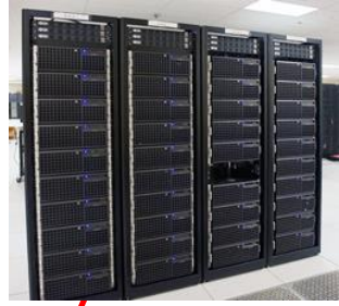
HPC Cluster Systems
