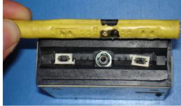
Cable after being "vampire" tapped.
